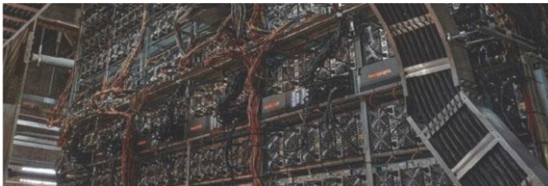
Bitcoin mining equipment installed within the Town of Torrey, NY mining facility.
